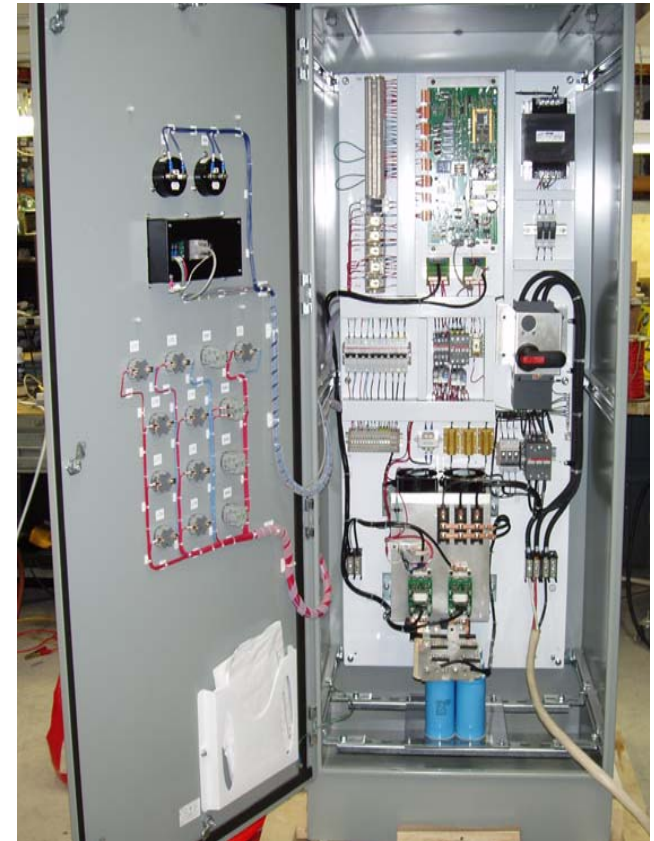
Mid Frequency 400Hz Power Supply Control Cabinet
