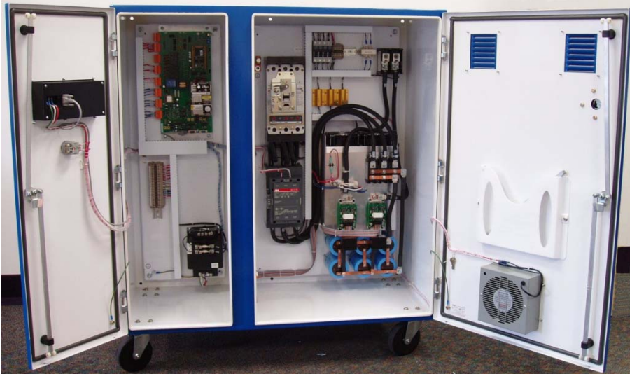
Mid Frequency 400 Hz Power Supply Control Cabinet
